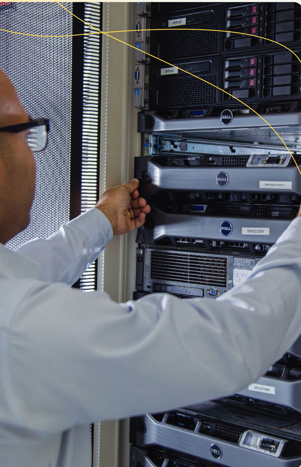
Data Center – Itumbiara (GO)
